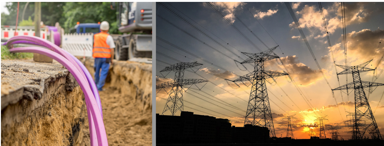
FIGURE 1 – Deployment of fiber cables in trenches (left) and overhead power lines including fiber cables (right)
